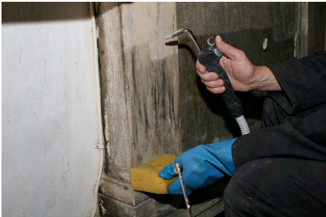
Steam cleaning of the left pilaster in progress, with dirty residues collected in sponges to prevent re-distribution.
