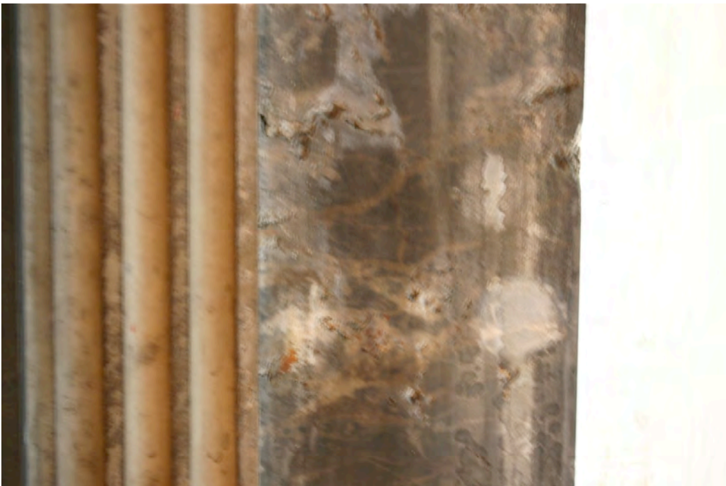
Detailed view of the poor (geological) quality of the light-grey decorative marble, with historic loss of material to the unusually weak calcite component. This is across the whole surface area of the slab and is not isolated to this area. Despite its dramatic appearance deterioration is not accelerated or progressive and these areas still remain solid. The deterioration may even be due to the original polishing process.
