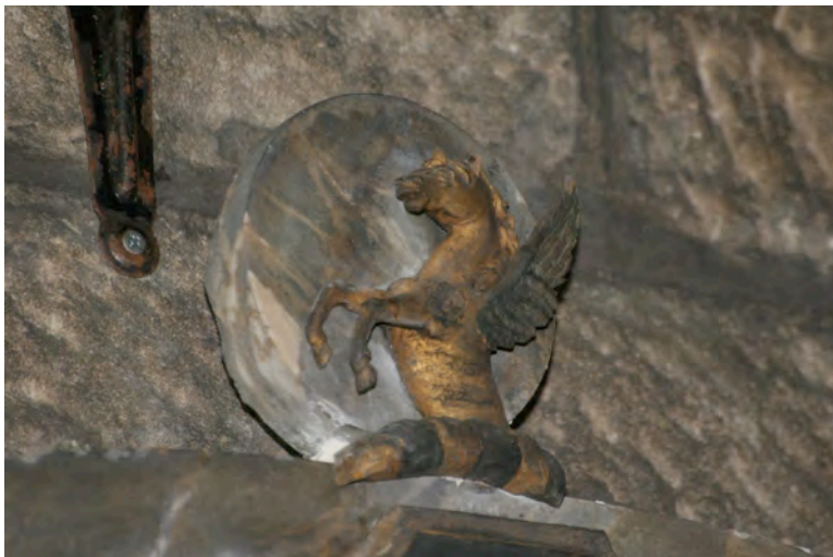
Detail of the winged horse and disc of marble behind, both having been removed, cleaned and re-secured.
