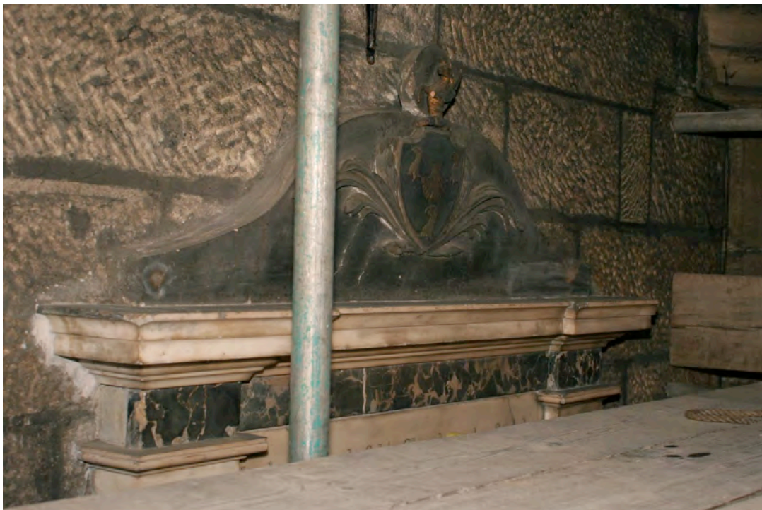
Detail of the pediment and cornice before treatments, note the curvilinear pediment looks like a dark-grey carboniferous limestone but is in fact a heavily veined marble the same as the pilasters. Note also the heraldic representation of the horse is completely lost despite being gilded. Despite looking attractive, the frieze highlights the weak nature of this 'metamorphic' rock with a poor (large) crystalline structure having cooled quickly when formed originally.
