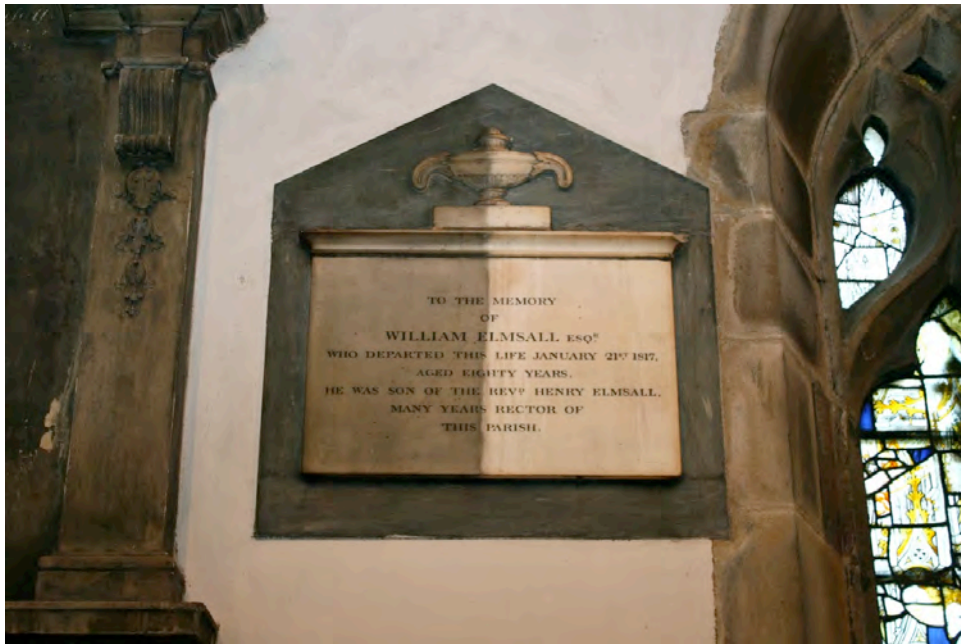
A cleaning contrast with signs of vertical water marking visible on the cleaned part of the inscription panel now.
