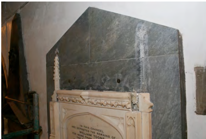
The background panel after cleaning with the loose pinnacle and bratishing removed for cleaning and re-attaching properly. Note the veining to the background marble is visible once again.
