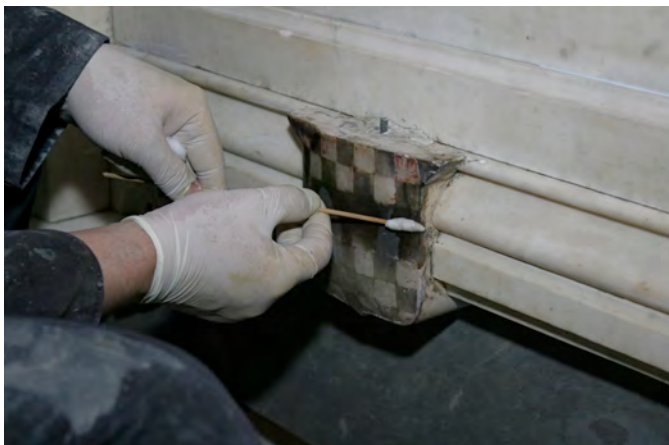
Cleaning the shield at the bottom of the monument, without disrupting the paint beneath.
